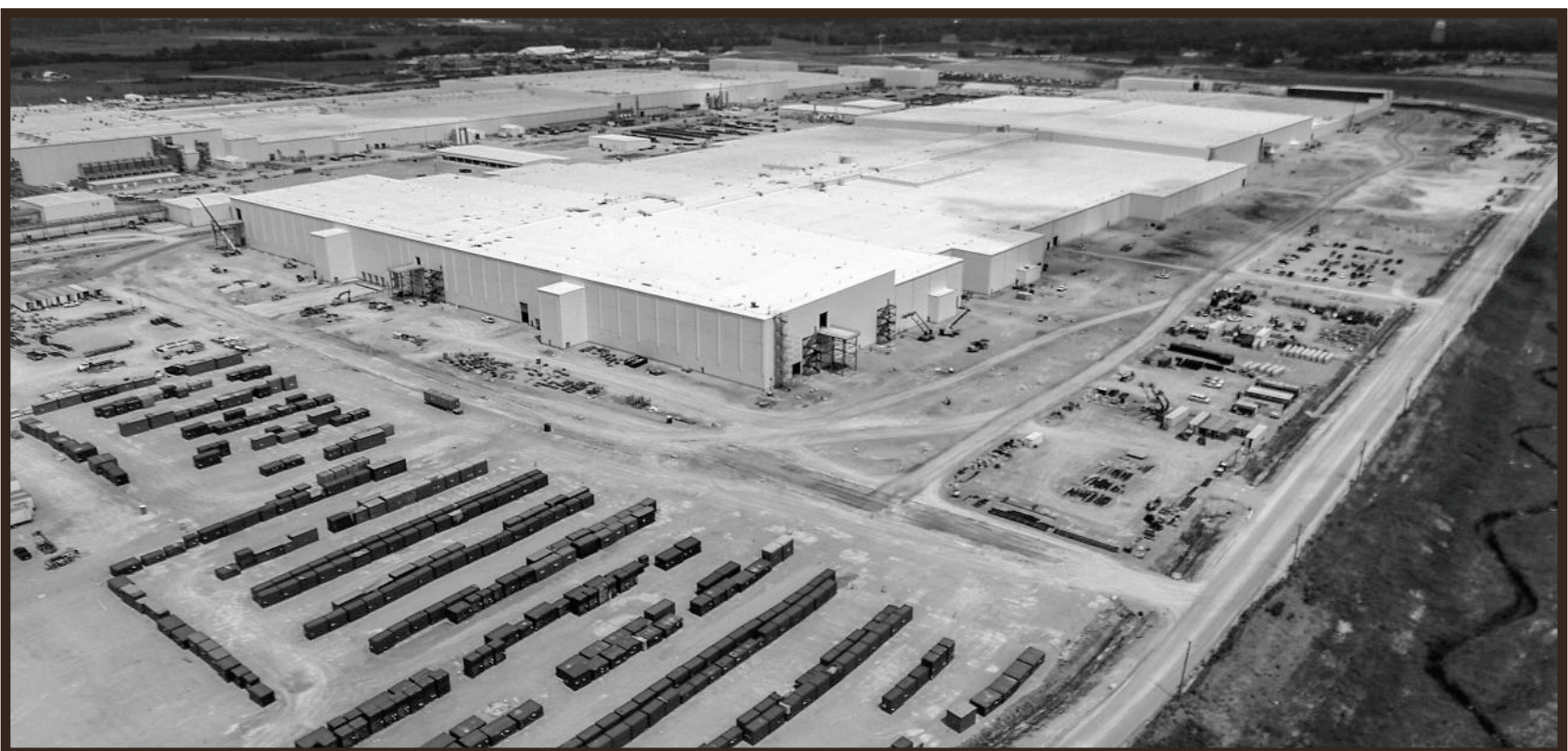
The Blue Oval SK Battery Park under construction in Glendale in July 2024. MICHAEL CLEVENGER AND SAM UPSHAW JR./COURIER JOURNAL
