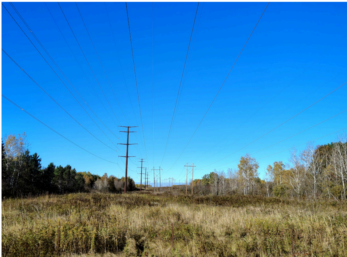
Minnesota Power transmission lines, Adolph. Credit: John Ramos
